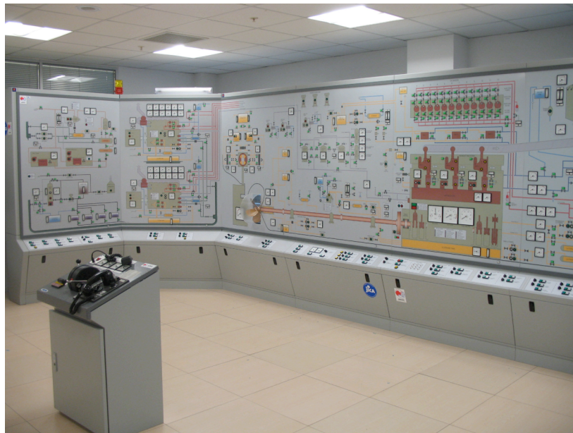
Fig. 2 The new mimic panel
