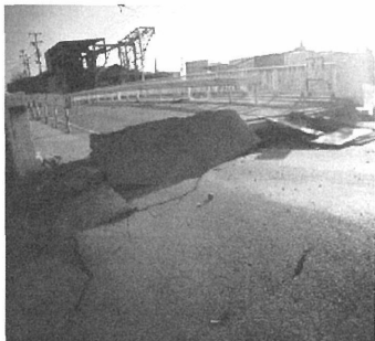
Fig.2.1 Damage situation of Karumo-Bridge drums 1,2)
