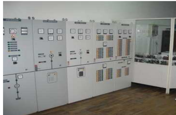
Figure 1 Main switch board
