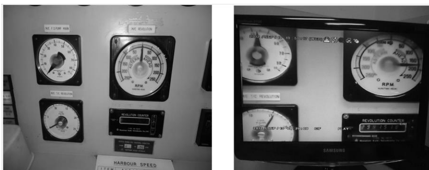
Figure 9 Operating parameters on main control box
