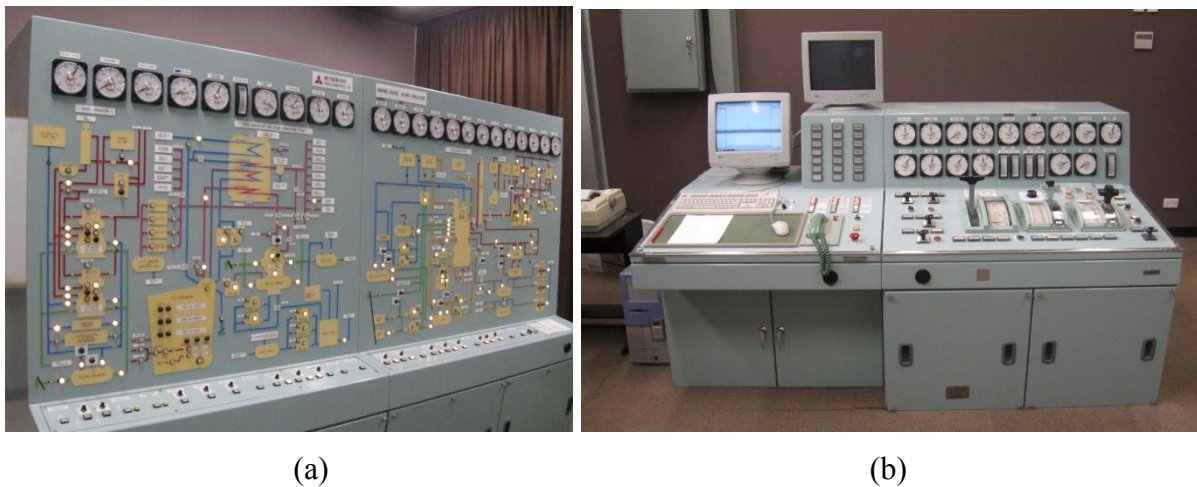
Figure 1. (a) Hardware based Engine Simulator installed at AMC in 1985, showing the entire engine room and the machinery space analogue mimic panel, (b) Engine Control Room console.
