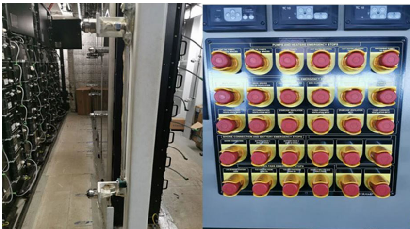
Figure 5 - The port side battery department and emergency stop console from the bridge - M/S AURORA BOTNIA (Source Heikki Koivisto)
